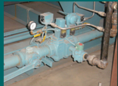
Biodiesel Steam Boiler
